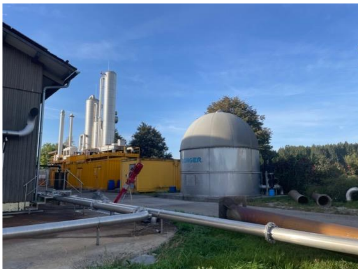
Photo 1 - Standing on top of the digesters looking at the gas upgrading plant
