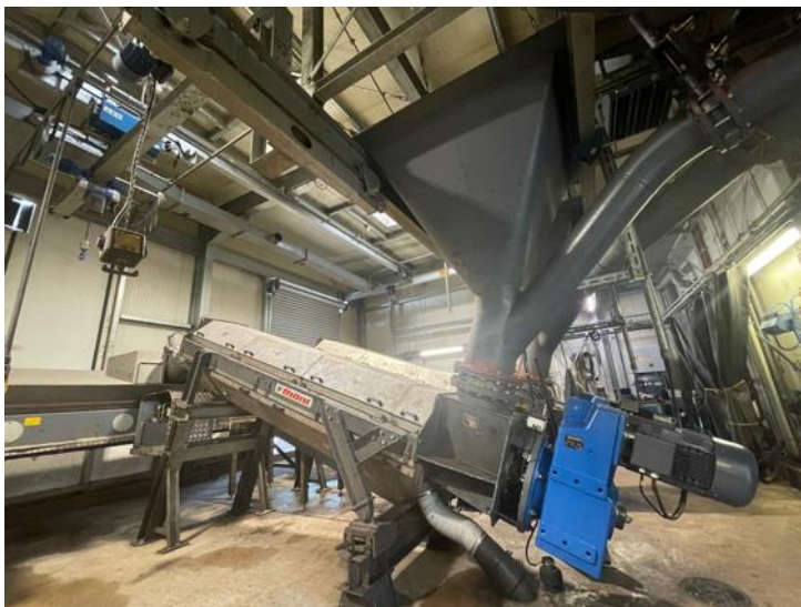
Photo 10 - Input to plug flow digesters
